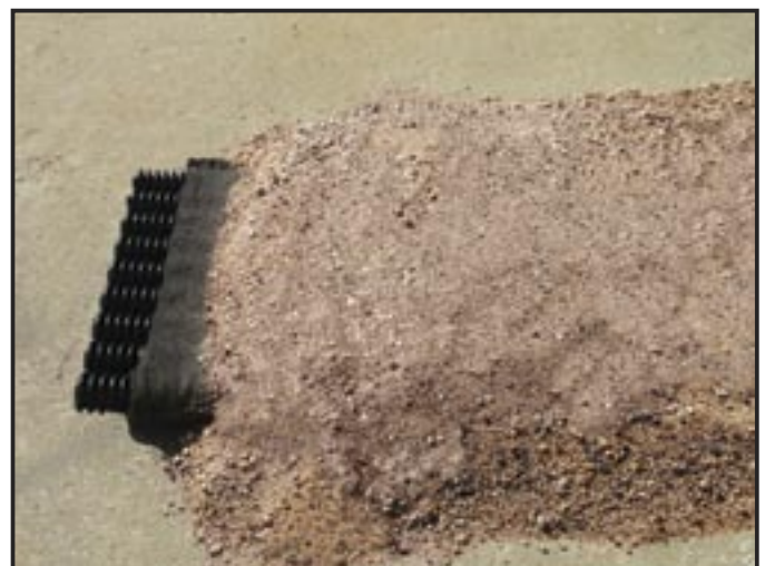
Clean, very coarse sand acts as an excellent filter, dramatically extending the life expectancy of the system. A 2 inch band should be installed covering the top and sides of each collector line.
