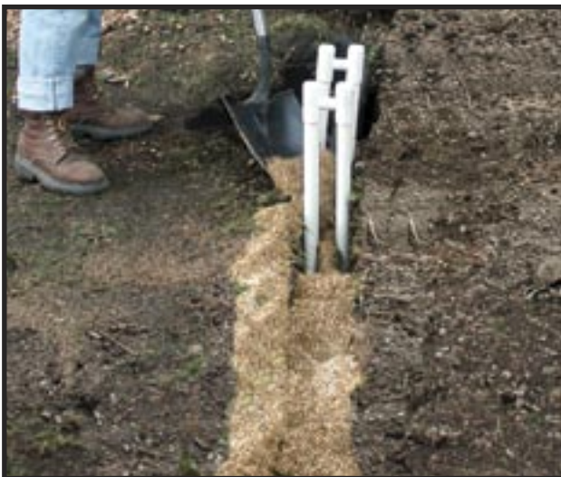
Centering devices are helpful for holding Multi-Flow in the middle of the trench while backfilling.
